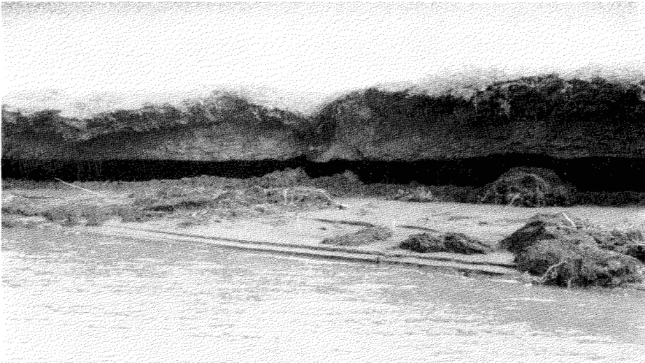
Fig. 3. Exposed undercut along right bank of the Colville River.
